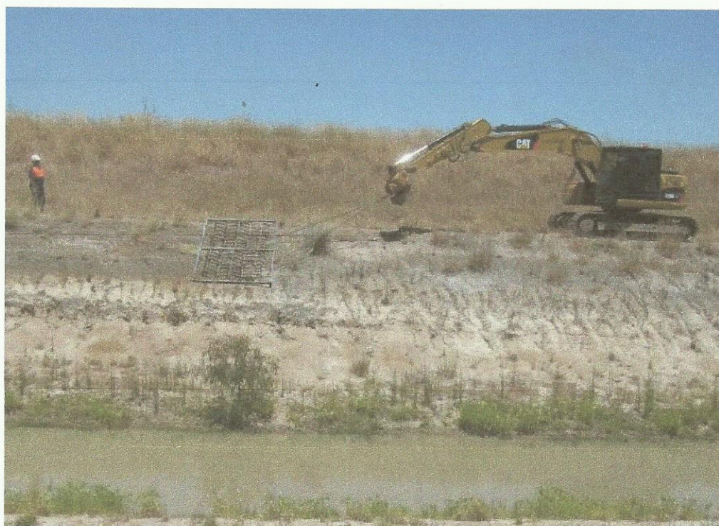
Figure 2. Excavator towing custom made harrows along the channel batter. The untreated area of channel can be observed in front of the harrows.
